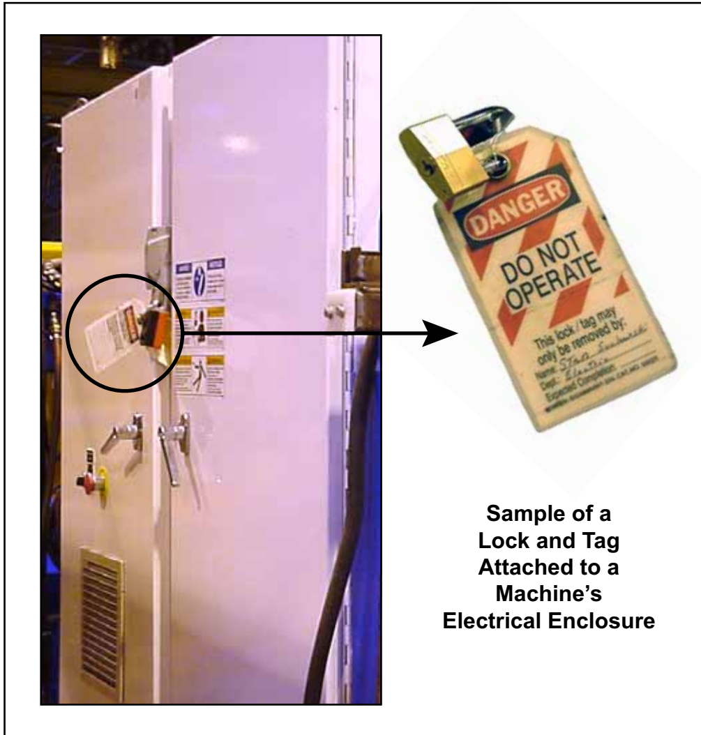
Figure 1: Lockout/Tagout on the Main Electrical Enclosure
